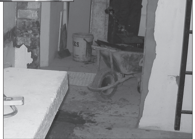
Photo by Khalid Salie Construction of new nutrition lab in South Africa
